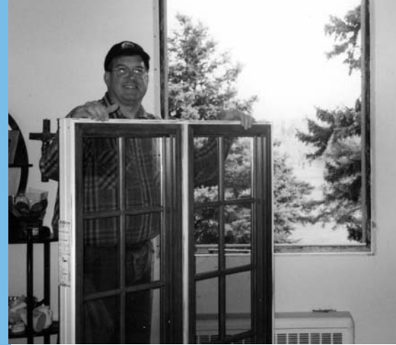
▶ John Stonefoot (Ground Maintenance) insures a seamless fit during the initial phase of the window replacement project.
